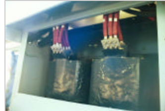
Above: Large DC link reactors used in 4160 volt 5000 hp VFD.
