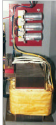
Left: Reactor used in conjunction with capacitors for harmonic filtering.
